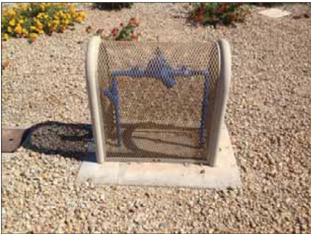
Backflow Preventer - multiple locations 13 total
