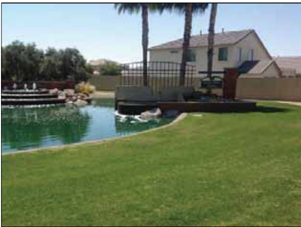
Water Feature multiple locations - Filter, Pump and Motor
