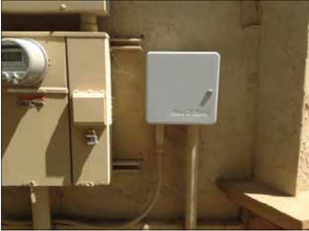
Rainbird Irrigation Station - multiple locations 26 total
