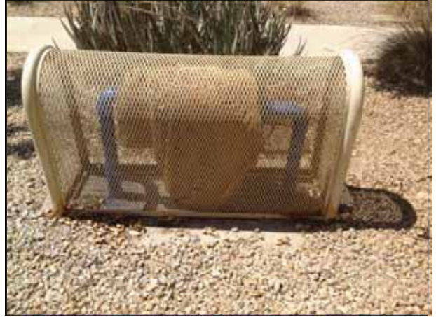
Backflow Preventer - multiple locations 13 total
