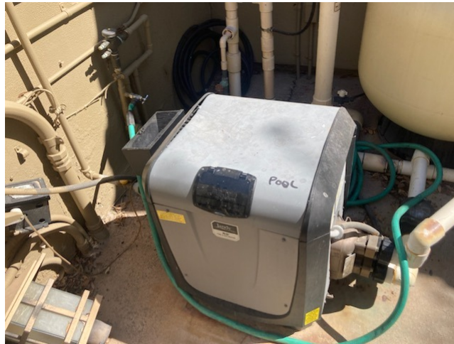
This is a Jandy pool heater. Was a Hayward heater in 2020.
