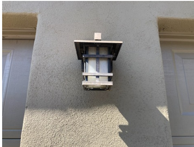
The wall mounted, lantern fixtures at the garage buildings were last replaced in 2007.
