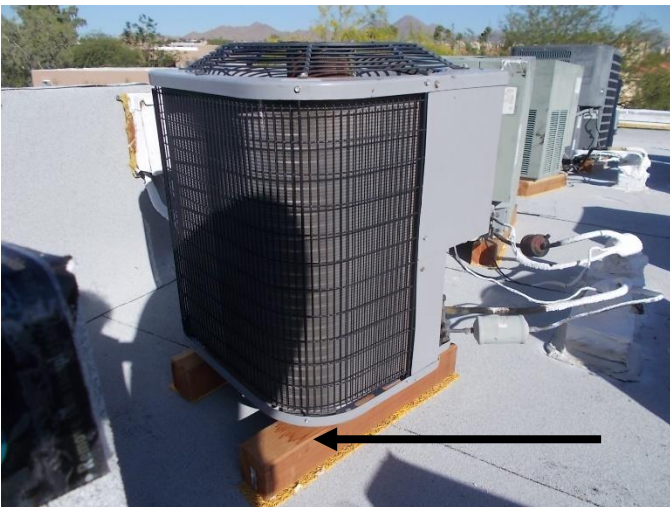
Do not disturb the existing wood support blocks and reuse if at all possible. Protective slip sheets should always be installed between the roof system and any type of equipment platform or support.
