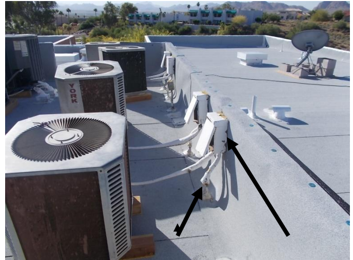
Take great care to seal around any roof penetrations that may be needed and/or any existing roof penetrations that are disturbed. Make sure the disconnect box is properly sealed around.
